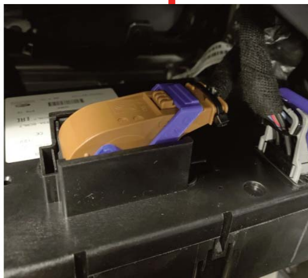
BCM Brown connector in rear of BCM/fuse box 60 pin plug. Rostra Red ignition wire connect to DK. Blue wire in position 12.
